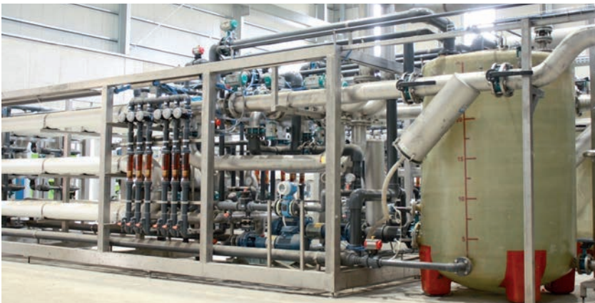
FIGURE 2. EXTERNAL MBR: UF SYSTEM WITH BERGHOF MEMBRANES MODULES
